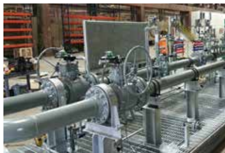
PROJECT: JHAL MAGSI GAS FIELD INTEGRATION PIPELINE
